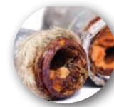
Internal Pipe Corrosion
